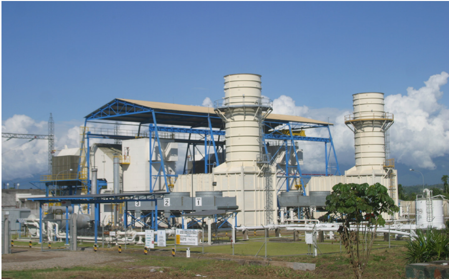
Duke Energy - Central termoelectrica de Aguaytia
