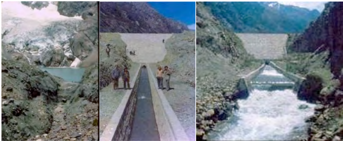
Constructing the Shallap Lake safety dam and water channel in 1973 and the completed work in 1974. Photos: César Portocarrero
