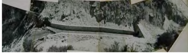
Safety works on Huallacocha Lake: 1950s construction (top) and the finished result in the 1960s. Photos: Glaciology Office Archives
