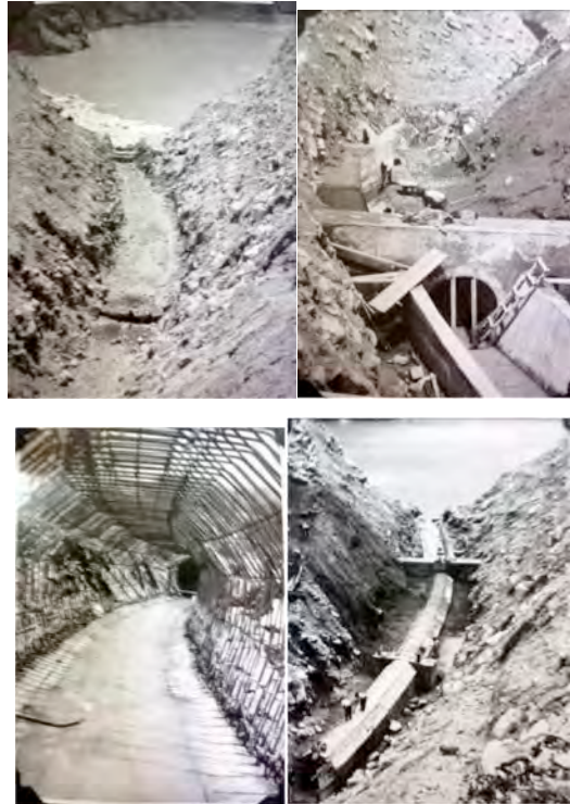
New tunnel being constructed in the early 1980s. First the channel was cut, then the tunnel built, and finally the canal was covered with a safety dam. Photos: César Portocarrero
