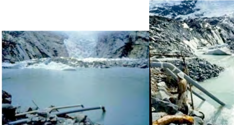
The initial siphoning process to lower the water level of Lake 513 in the late 1980s. Siphoning was an interim measure until funding was received for construction of the tunnel. Photos: César Portocarrero
